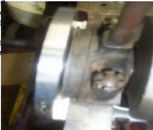
Now with this all aligned and torqued it is time to add the sealant.
